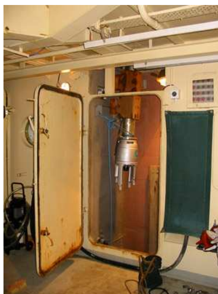
Figure 22 – GAPS inside a hoisting pool
